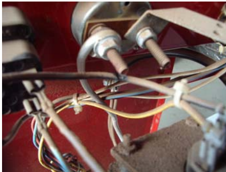
Wire in contact with bolt allowing 240-volt ac to the positive lead and clamp
